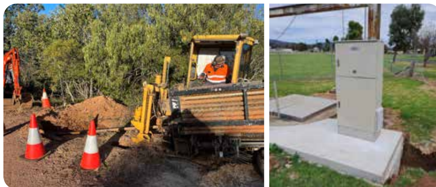
Below: Horizontal drill installing pressure sewer pipes. Right: New electrical switchboard at pump station 3, Bingara
