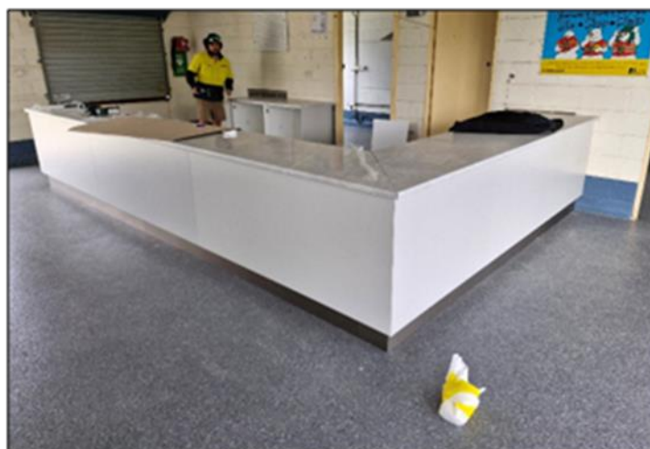
New counter installed at Warialda Swimming Pool
