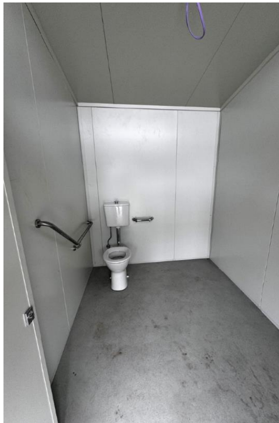
Warialda Rail Recreation Ground accessible toilet
