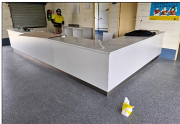
New counter installed at Warialda Swimming Pool
