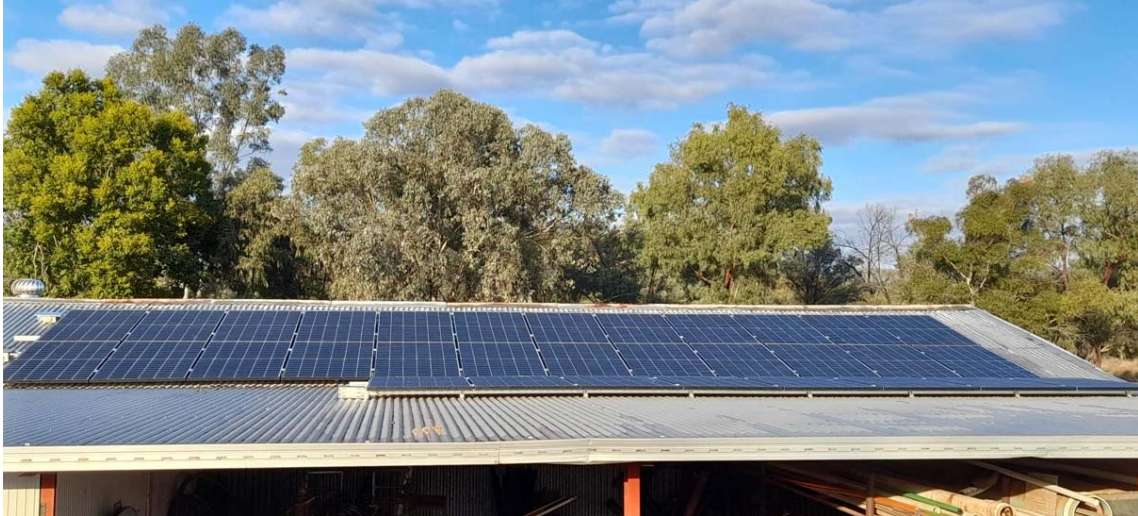
New solar panels on the roof of the Sewerage Treatment Plant, Bingara
