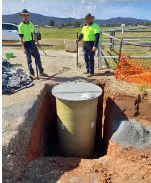
The pump station at the new amenities block at Bingara Showground
