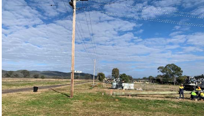
The electrical infrastructure is being completely installed at the Bingara residential subdivisions.
