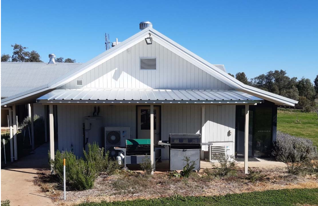
The Building Crew have completed the extension on the eastern side of the Classroom to provide a cover over the BBQ area.
