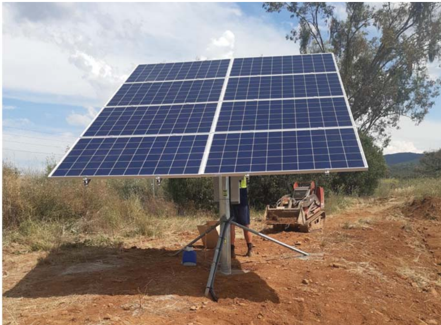
New solar panels at Bingara Sewerage Treatment Plant
