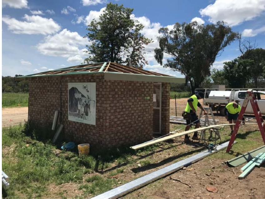
Warialda Saleyards amenities – repairs being undertaken after a tree fell on the building
