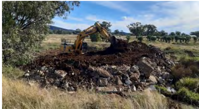
Broken concrete from the Bingara swimming pool
