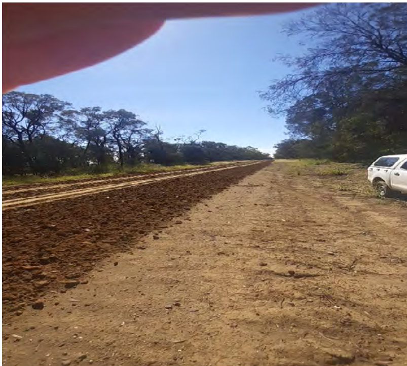
SR41 County Boundy – Trial of Polycom, which is a road stabilising additive
