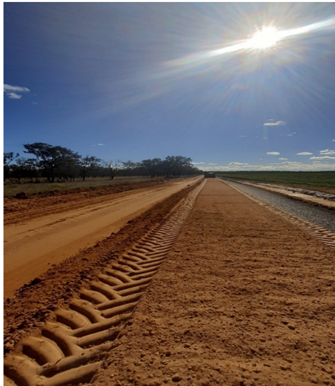
North Star Road – Flaggy, Stabilising
