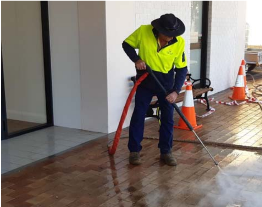
Cleaning in front of the new library in Maitland Street, Bingara with the steam weeder.
