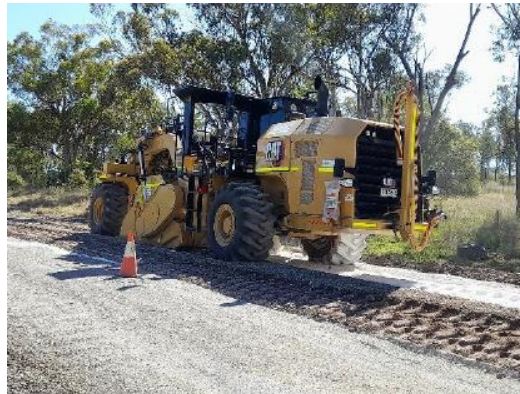
Heavy Patching, Fossickers Way
