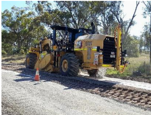
Heavy Patching, Fossickers Way
