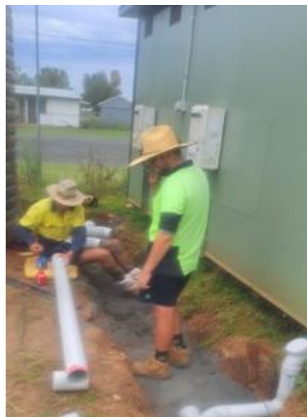
Upper Horton Amenities Plumbing
