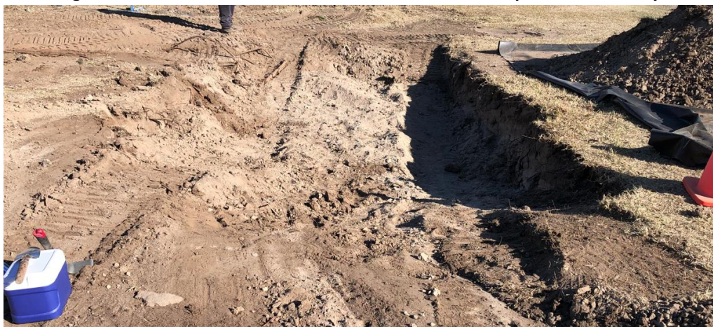
Figure 6: Fuel tank was located in northwest sector of Respite Centre facility.
