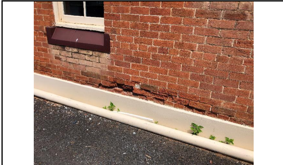
Photograph 11: Shows damage to the brick walls above the DPC.
