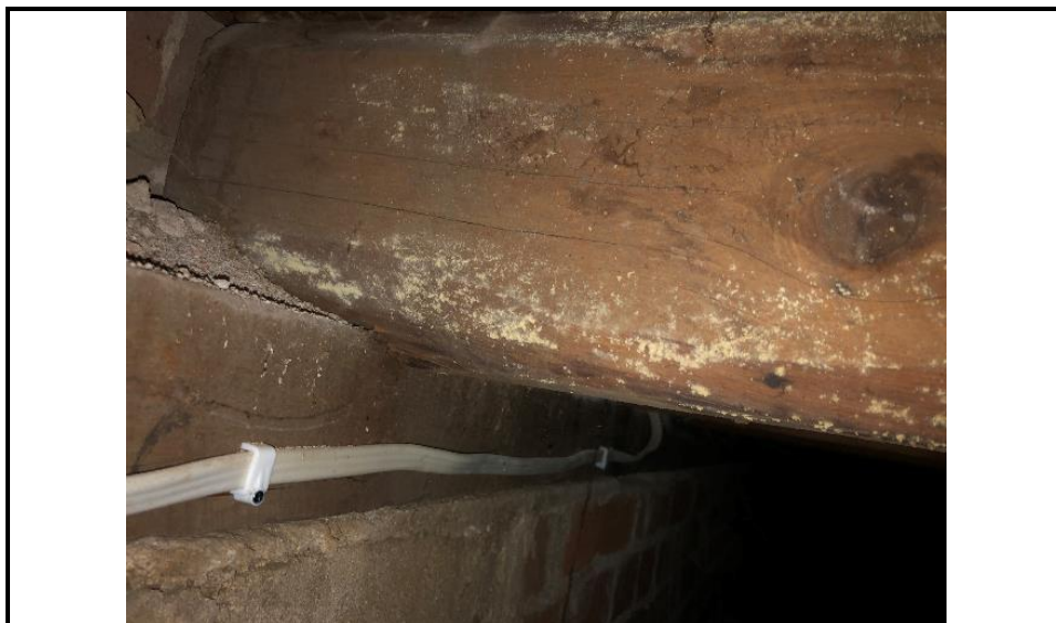
Photograph 40: Shows mould to the floor frame under the original section.
