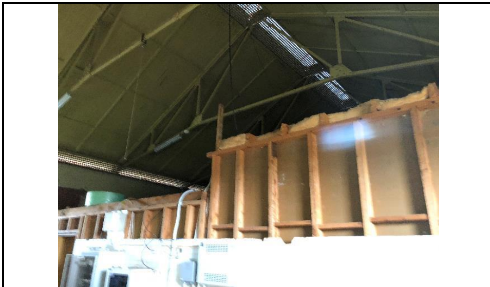
Photograph 36: Shows the office fit out to the Town Hall section of the original building.
