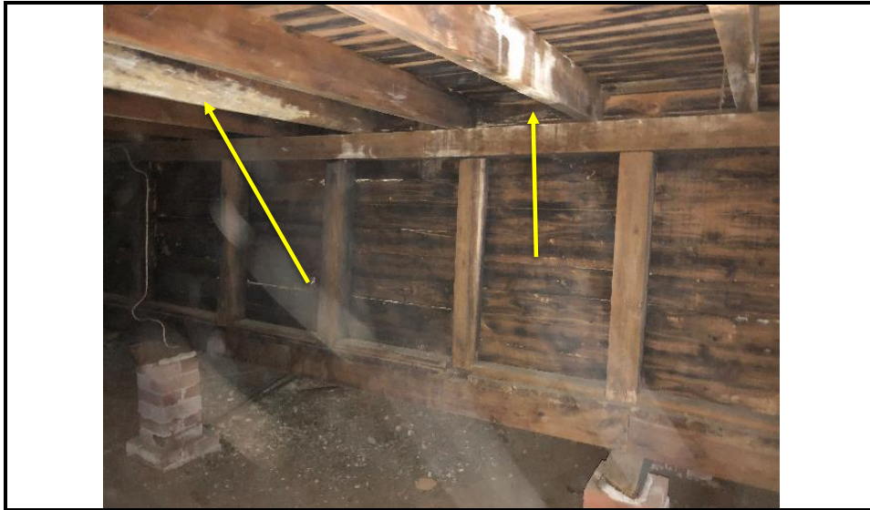
Photograph 33: Shows mould to the floor frame.
