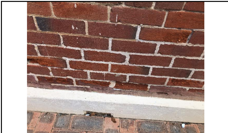
Photograph 4: Shows the wall vent under the pavers and where the bricks and mortar have been patched previously.
