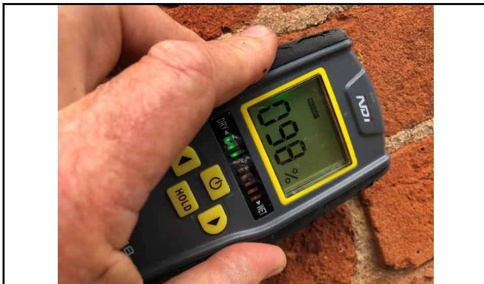
Photograph 12: Shows the raised moisture levels above the DPC.
