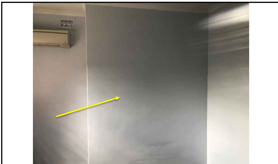
Photograph 30: Shows the affected wall in the Back Office.
