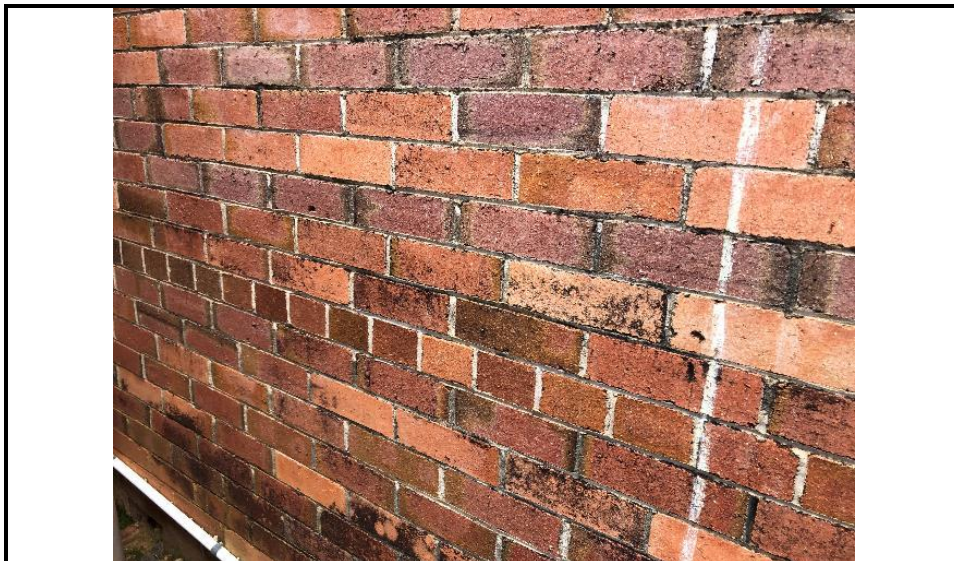
Photograph 22: Shows mould to the external brick wall outside the Rear Entry Office.
