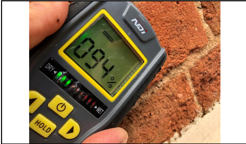
Photograph 13: Shows the raised moisture levels above the DPC.
