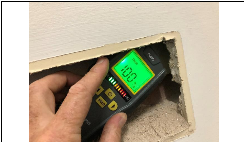
Photograph 38: Shows the moisture level to the existing external brick walls behind the office fit out.
