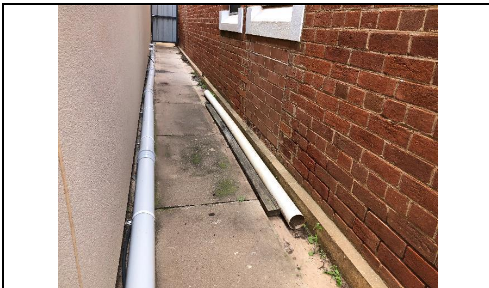
Photograph 16: Shows the western end of the southern wall elevation where all the wall vents have been covered.
