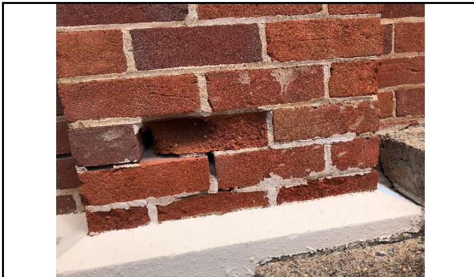
Photograph 10: Shows damage to the brick walls above the DPC.
