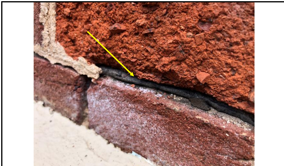
Photograph 8: Shows the fretting to the bricks above the DPC.
