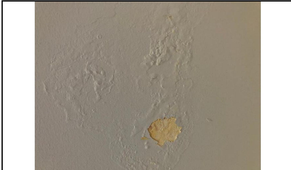
Photograph 27: Shows water damage to the southern wall.
