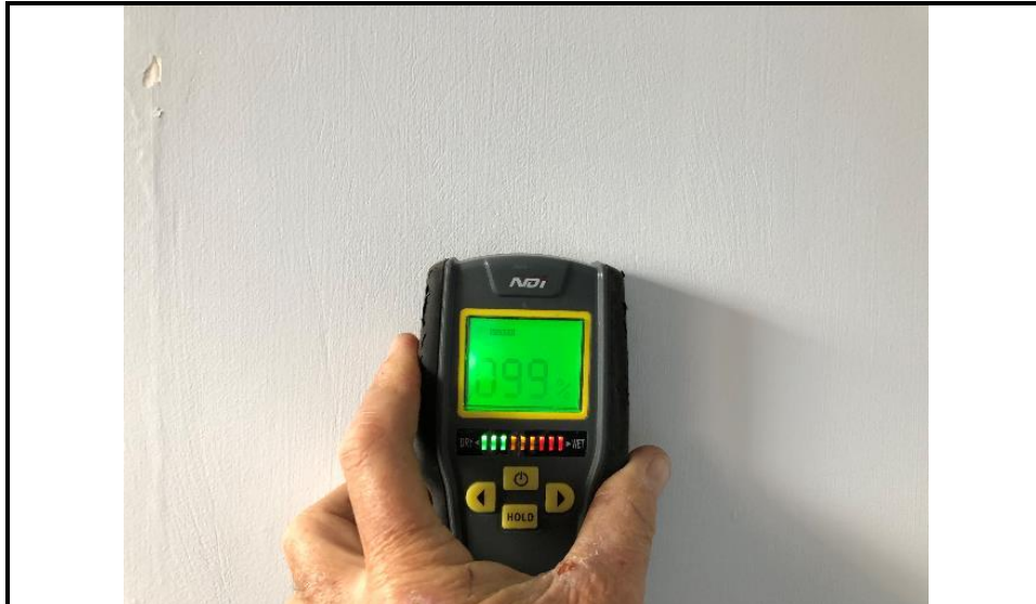
Photograph 31: Shows the moisture level to the affected wall in the Back Office.
