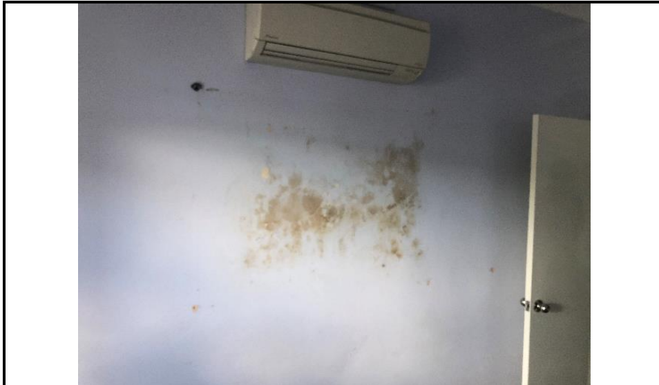
Photograph 25: Shows mould to the southern wall.
