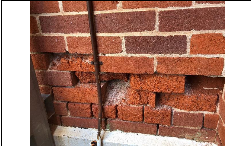
Photograph 17: Shows damage above the DPC to the southern elevation.
