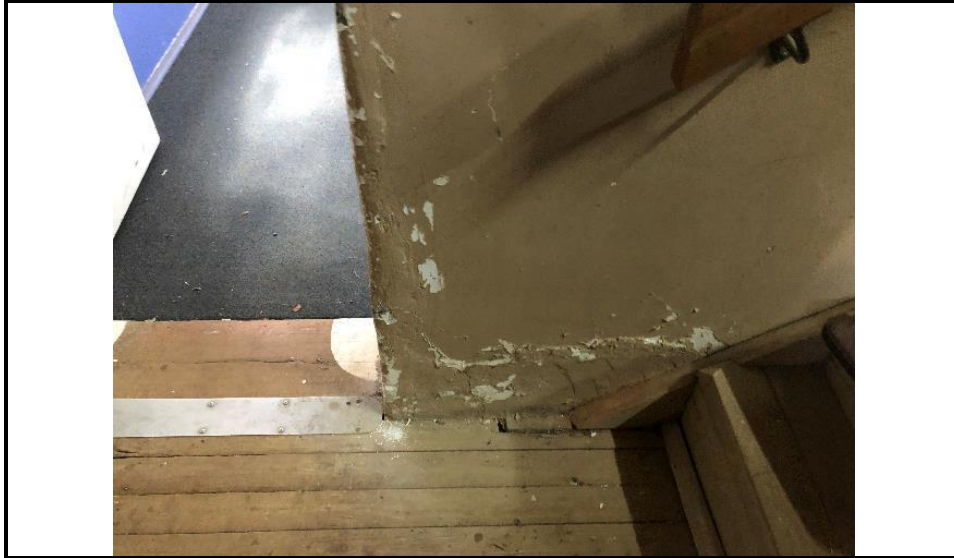
Photograph 35: Shows rising damp damage near the access hole to the sub-floor area.
