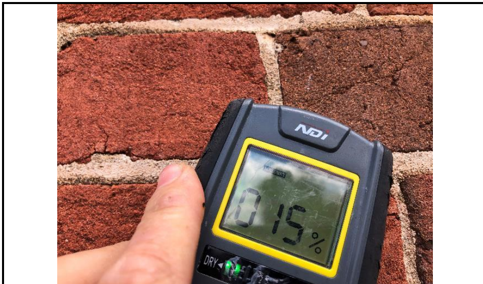
Photograph 14: Shows the moisture levels further high up the wall.
