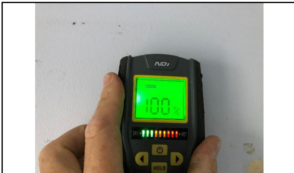
Photograph 28: Shows the moisture levels to the southern wall.
