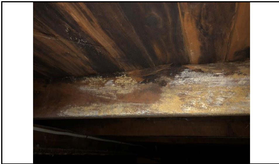
Photograph 34: Shows mould to the floor frame.
