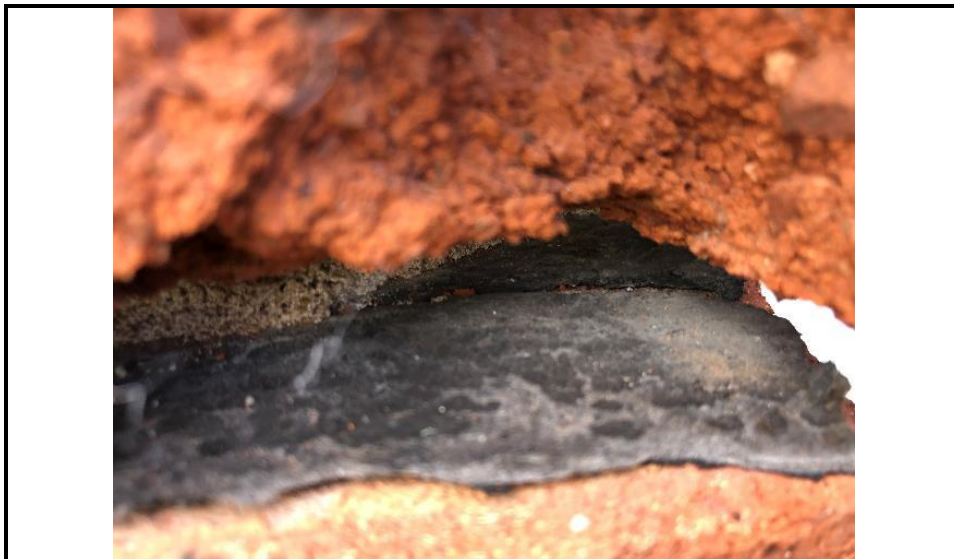
Photograph 20: Shows the DPC and a damaged brick above.
