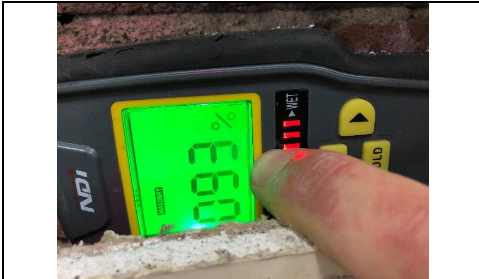
Photograph 39: Shows the moisture level to the existing external brick walls behind the office fit out.
