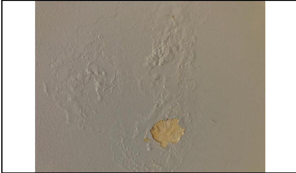
Photograph 27: Shows water damage to the southern wall.
