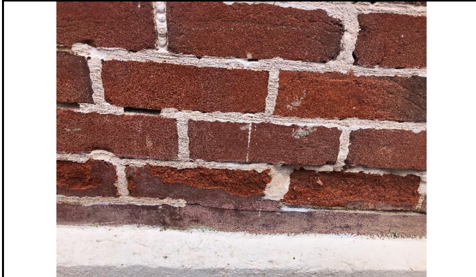
Photograph 5: Shows where the bricks and mortar have been patched previously.
