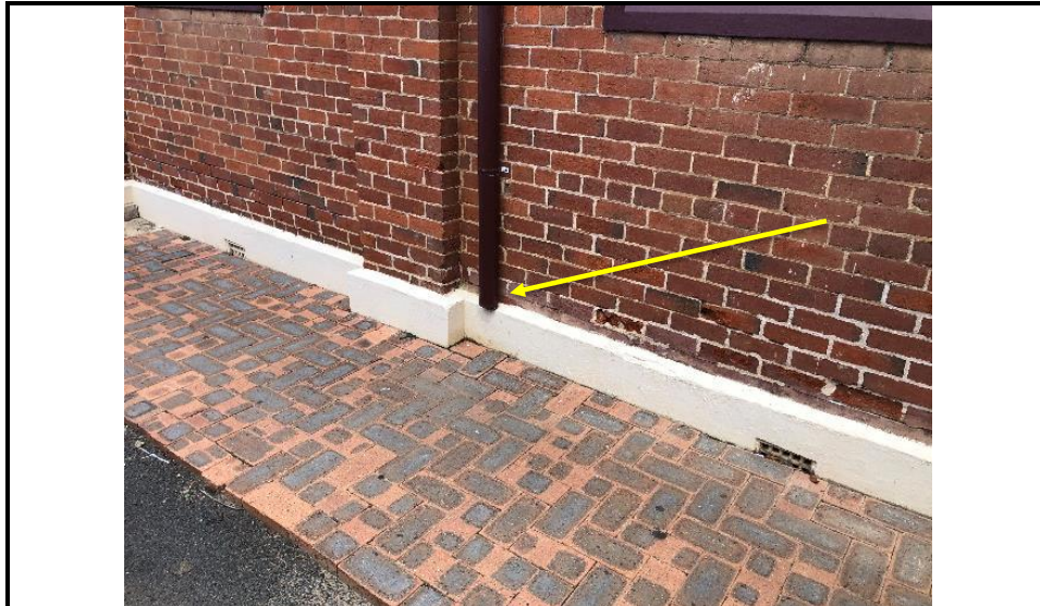
Photograph 7: Shows where a downpipe is discharging directly onto the ground.
