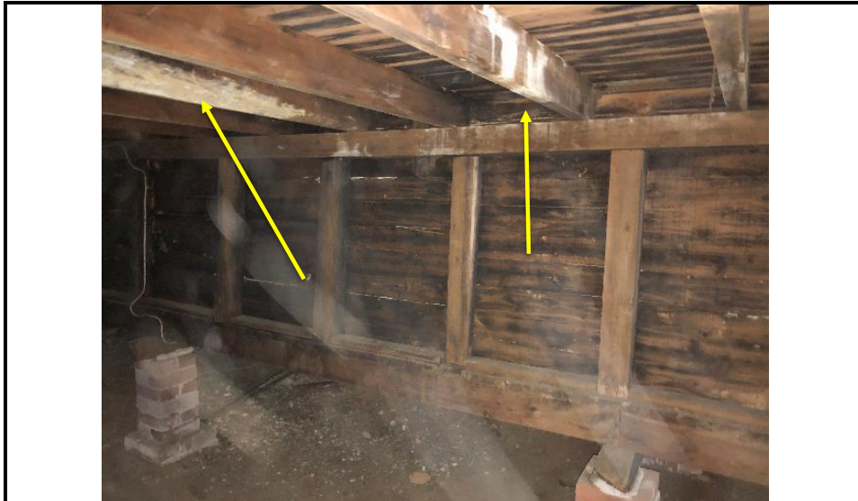
Photograph 33: Shows mould to the floor frame.
