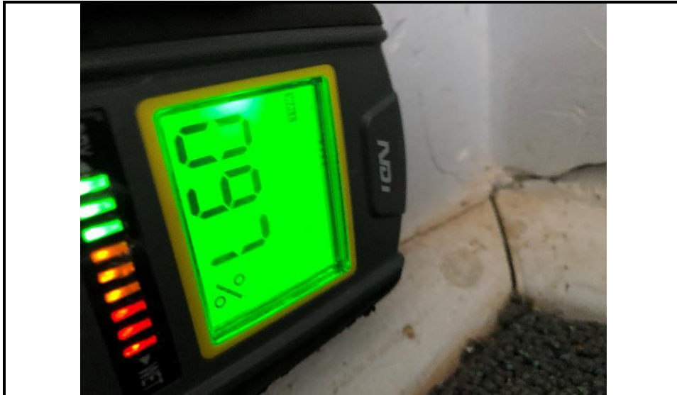
Photograph 29: Shows the moisture level to the northeast corner that adjoins the Back Office.
