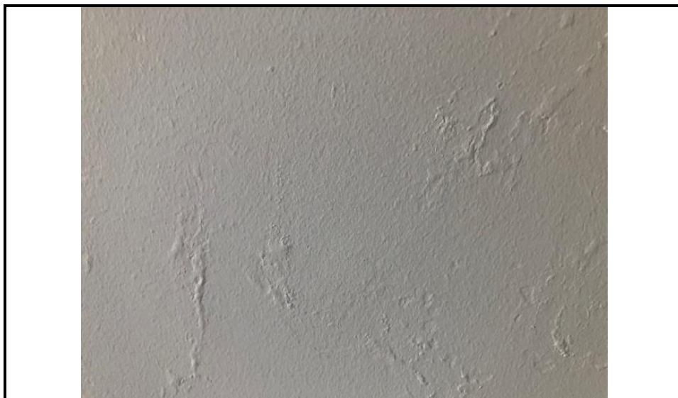
Photograph 26: Shows water damage to the southern wall.
