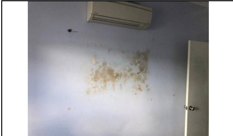
Photograph 25: Shows mould to the southern wall.
