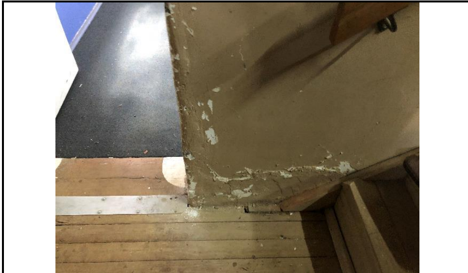
Photograph 35: Shows rising damp damage near the access hole to the sub-floor area.
