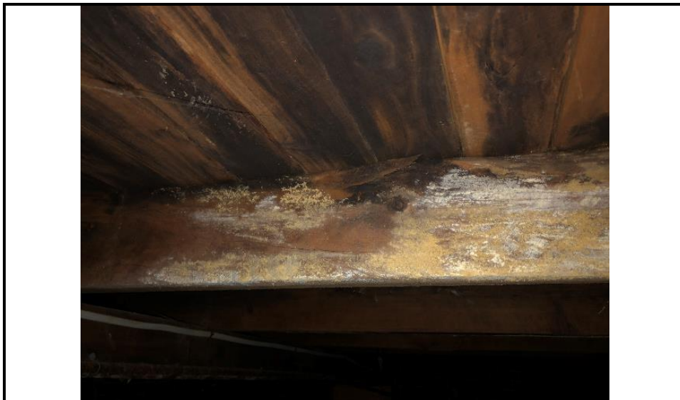
Photograph 34: Shows mould to the floor frame.
