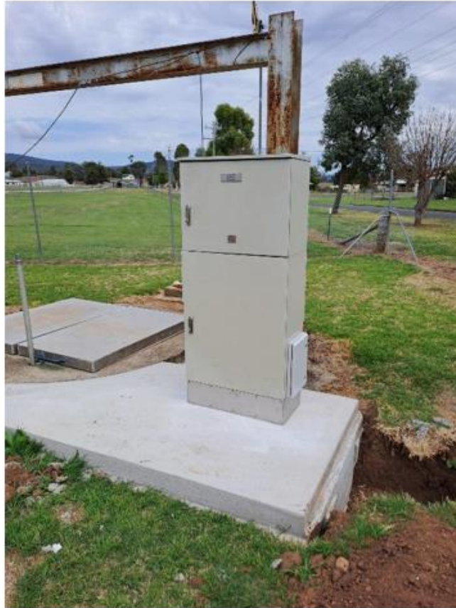
New power box PS3, Bingara
